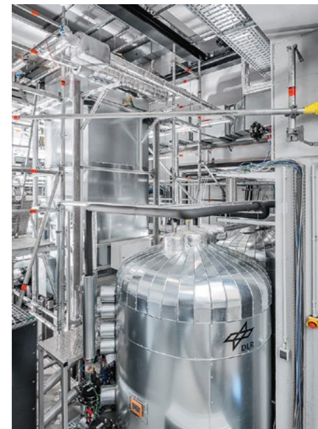
Carnot batteries store electricity in the form of heat. DLR and the CHESTER consortium (Compressed Heat Energy Storage for Energy from Renewable sources) are constructing the world's first Carnot battery based on steam power processes.
